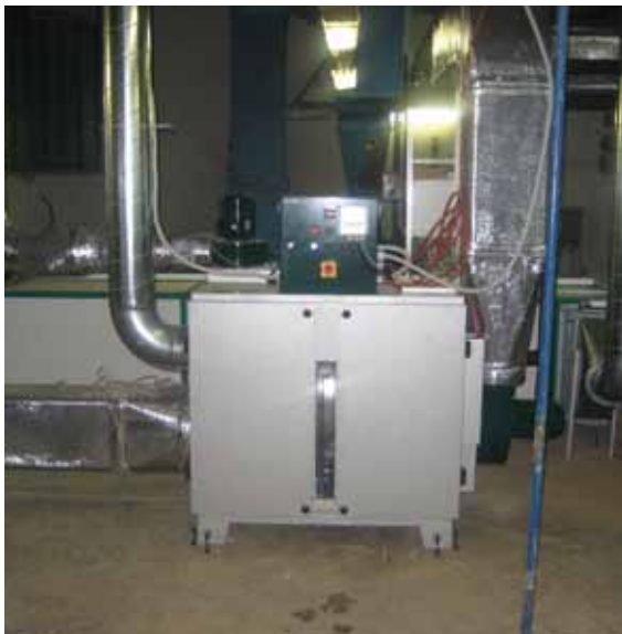
Installed RZ-071 unit with EH-3 control at MILEX cheese factory, Slovakia.
